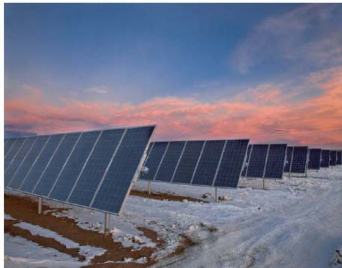
Hooper Colorado, Photo Courtesy of Array Technologies
